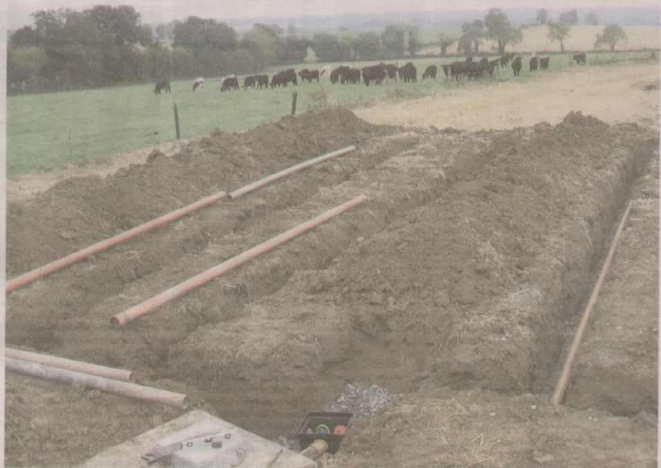
IN THE TRENCHES: Above is the bigger area of the percolation area with 18m long trenches fed from a distribution box. The pipes from this box are 4in/100mm perforated pipes that are laid with a slight fall over a bed of stone. The effluent from the tank flows by gravity from the tank as it fills up, firstly through the distribution box and then out through each of the pipes and into the percolation area by way of small 4-6mm holes at the bottom of the pipes
