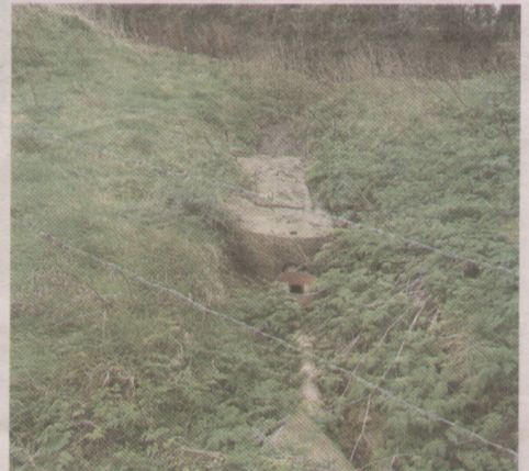
POOR DESIGN: This septic tank is a typical example of a badly designed system that is unfortunately all too commonly found in Ireland, according to Diarmuid O'Reilly of O'Reilly Oakstown Environmental. While the tank appears to be OK, there is an uncovered access point and the percolation area is an open sewer that leads directly to a drain 5m away under the trees. This drain connects to the local stream, river and eventually the sea and highlights the health risk the tank poses
